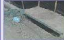
Failed Inlet Protection
