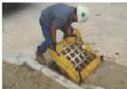
Replace SiltSack® and grate inlet into recess.
