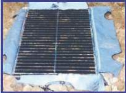
Installed Siltsack held in place by grate.
