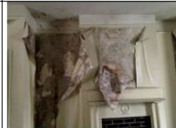
Deterioration of plaster
