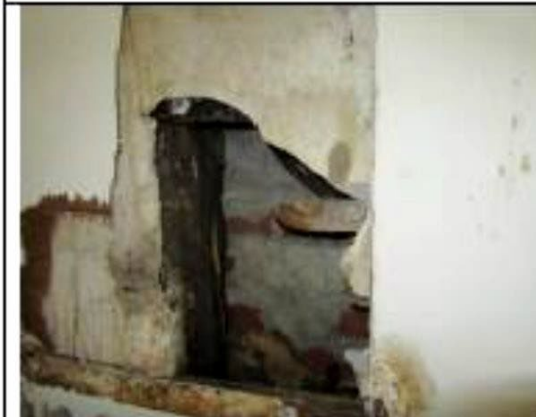
Deterioration of Wood Studs and Sheathing
