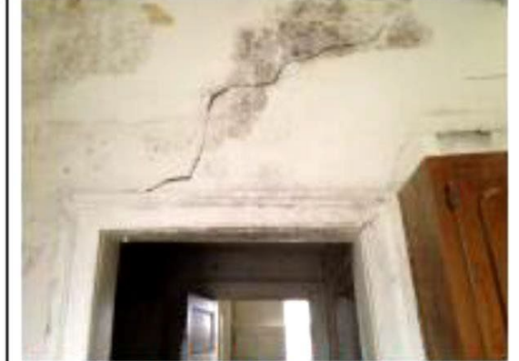
Extensive settlement from floor framing collapse
