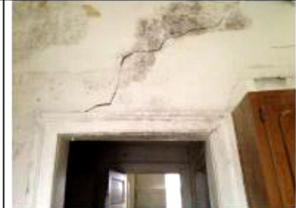
Extensive settlement from floor framing collapse
