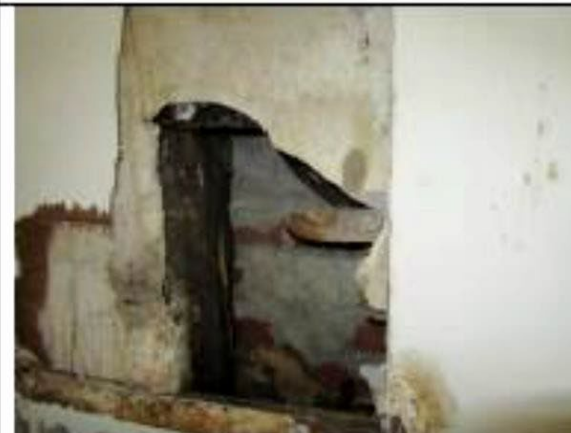
Deterioration of Wood Studs and Sheathing
