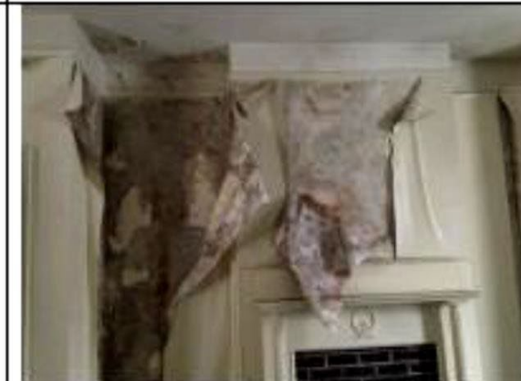
Deterioration of plaster
