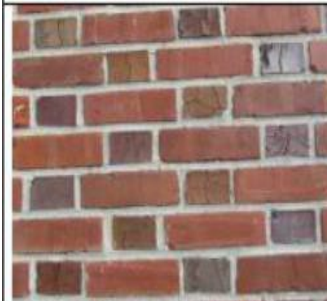
Extensive deterioration of Brick Shell allows water migration through wall. Spalling imminent.
